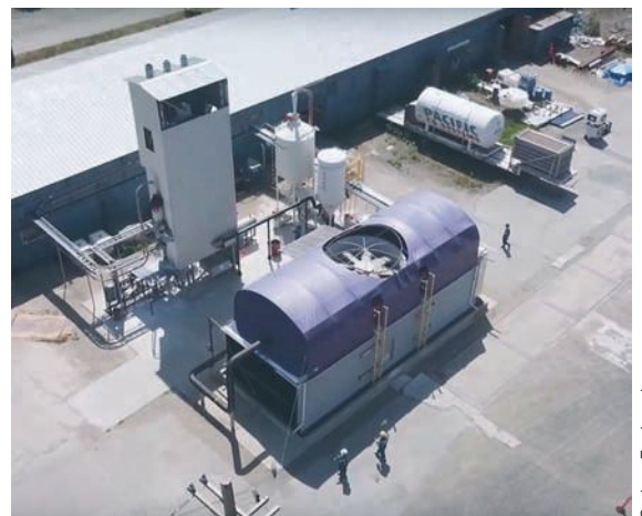
Photo 2—The giant fan in the center of the air contactor sucks in the air so other parts of the facility can separate out the CO 2 for processing into synthetic fuels.
