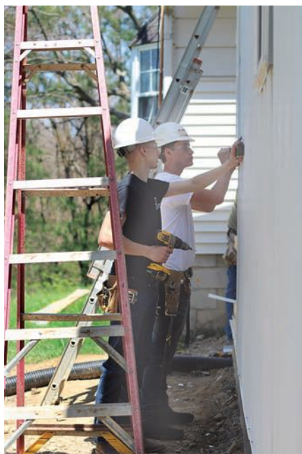
Students ensure that the siding is level at their 2018 project site in March. The group built a 24' x24' pole barn.
